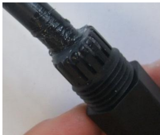
Figure 45 Cable Exit Area
